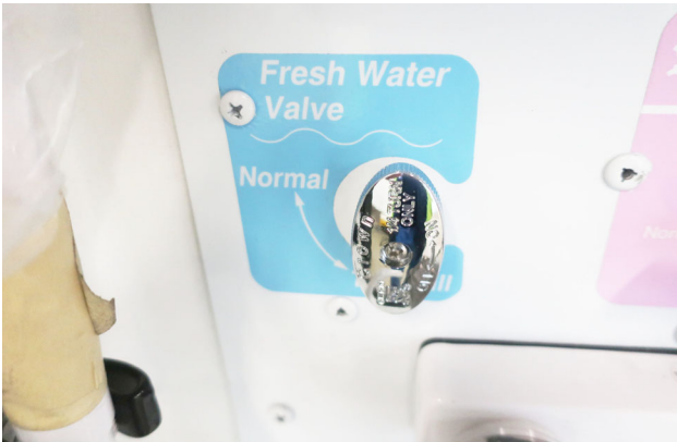
Fresh Water Valve (Located in water service center) -Typical View
