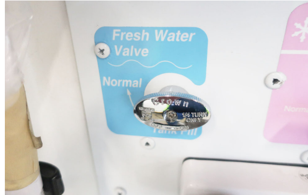
Fresh Water Valve (Located in water service center) -Typical View
