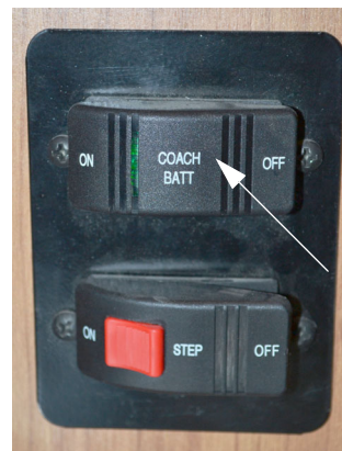
House/Coach Battery Disconnect Switch (Located near entrance door or end of galley, depending on model) -Typical View
